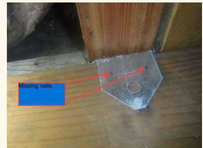
Missing nails in bracket.
