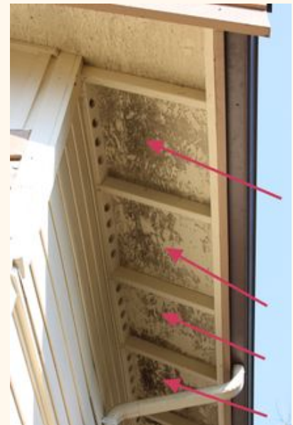
Examples of mildew on eaves.
