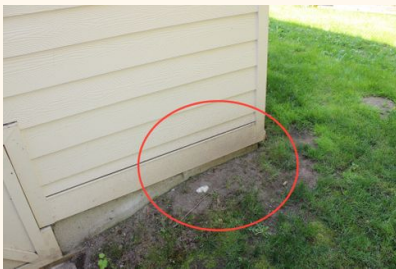
Less than 6" clearance to soil.
