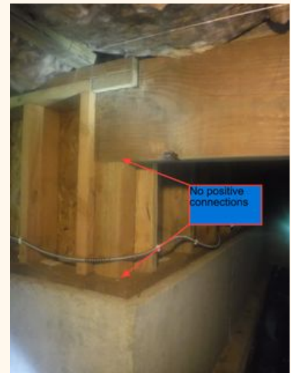
No positive connections between posts and footings.
