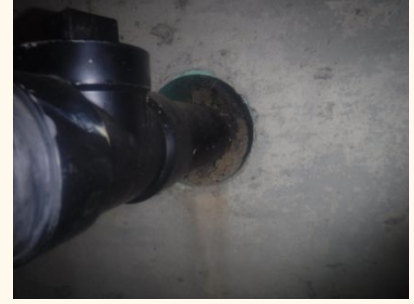
Sewer line not sleeved through foundation.
