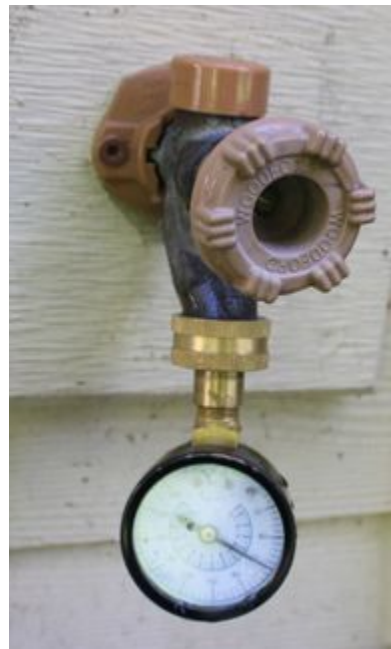
Hose bib rear of house.
