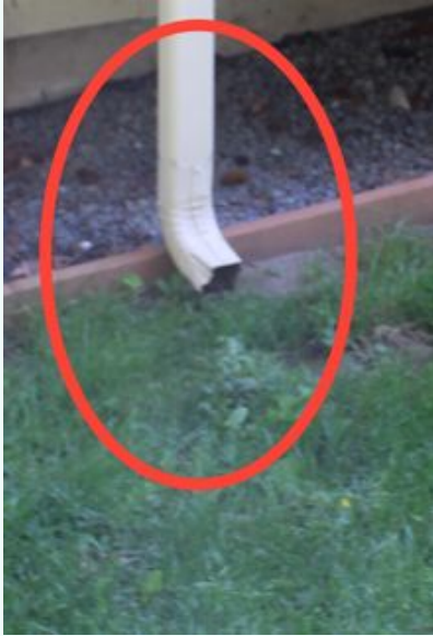
Downspout draining into yard.
