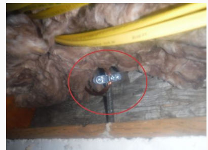
UFER ground under house.
