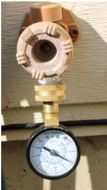
Hose bib front of house.
