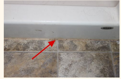
Caulking between bath tub and floor
