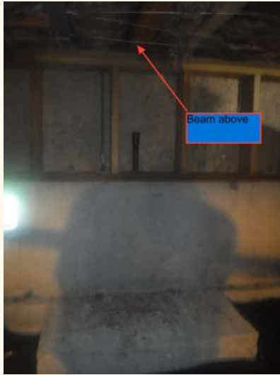
Beams not properly supported.
