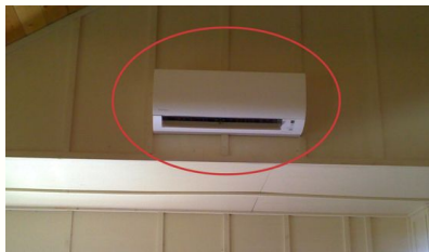
Heat pump indoor unit.
