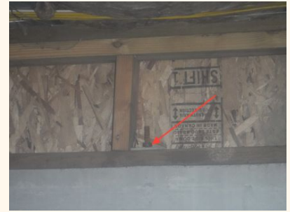
Loose nuts on foundation bolts.
