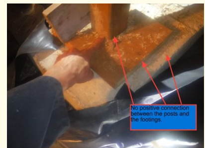
No positive connections between posts and footings.
