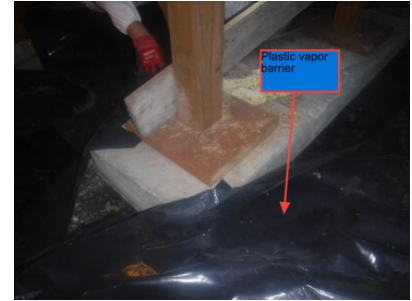
Plastic vapor barrier in crawl space.
