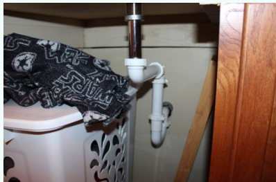
Waste line for bathroom sink.
