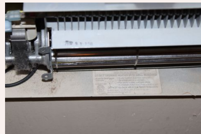
Typical dust in electric wall heater.
