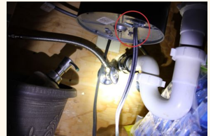
Garbage disposal under kitchen sink.
