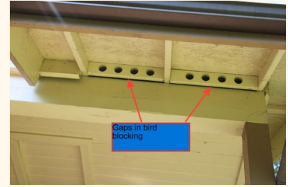
Examples of repairs needed to bird blocking.
