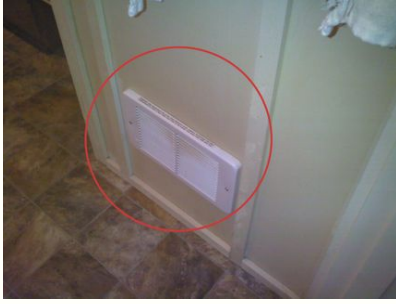
Electric wall heater.
