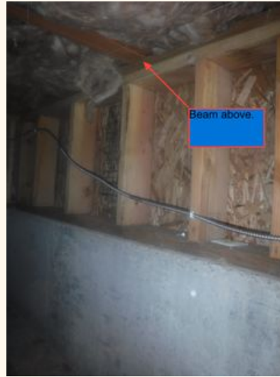
Beams not properly supported.
