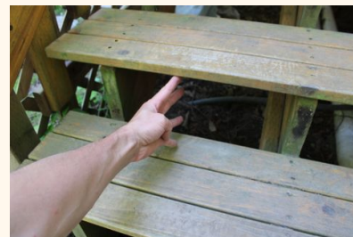
Openings between stair treads more than 4".
