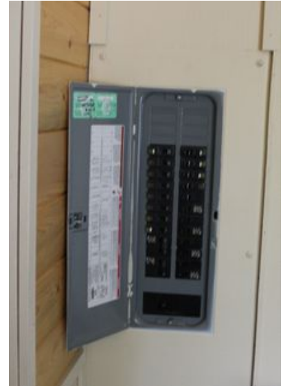
main electrical panel in front bedroom.
